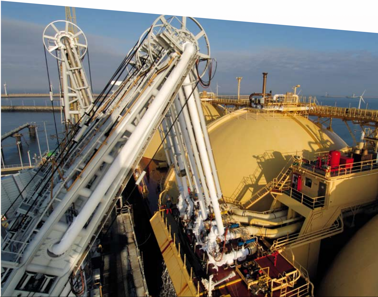
The LNG terminal in Zeebrugge saw a particularly high level of activity in 2009 with 78 ships unloaded.
